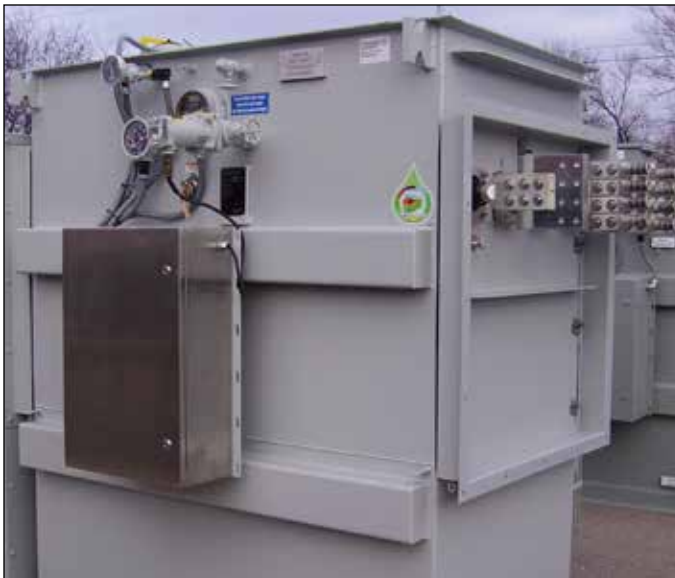
Figure 14. Substation transformer with customer-specific coordination and accessories.
