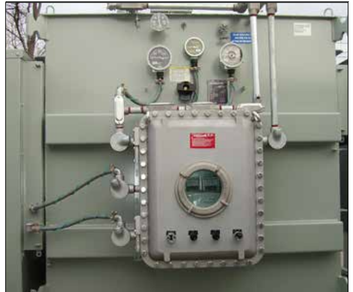
Figure 16. Class 1 Div 2 hazardous duty substation transformer.
