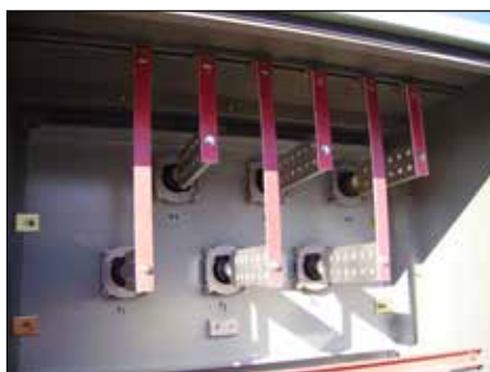
Figure 12. 12-pulse application with bushing supports.
